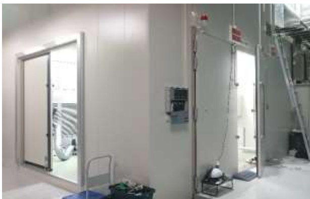
Fig.3.4.2-3 Outdoor unit room exterior
